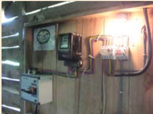
Illustration 6.19: The MFP in Leguruki provides off-grid rural electrification.
